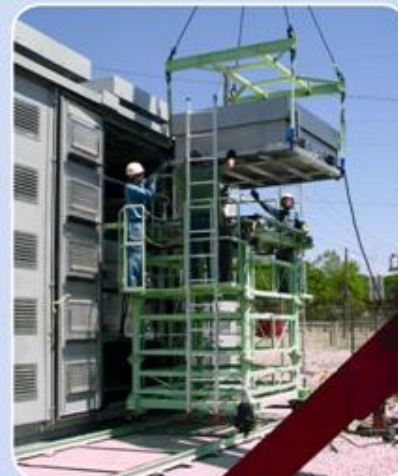
Lifting a battery module into place Photo courtesy of S&C Electric Company
